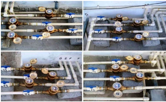
Fig 1 Complicated Networks of the Pipes
