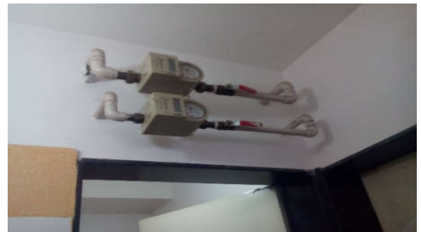
Fig 2 Well Planned Metering System
