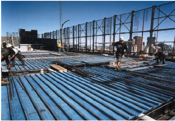
Fig 2 Composite floor, in construction for a high rise office and residential complex
